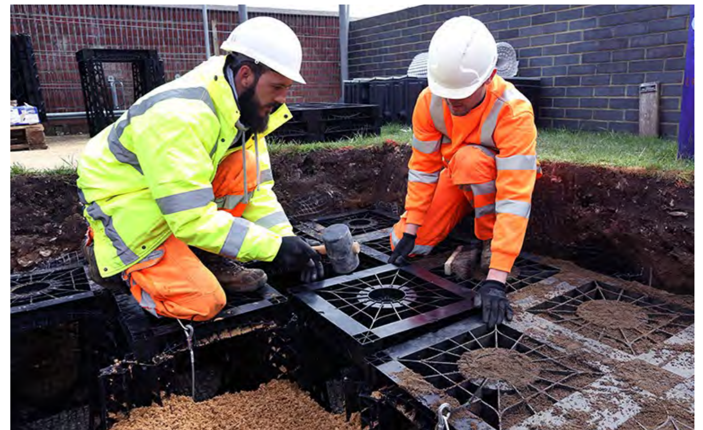
Creating a rainwater garden using sustainable drainage at All Saints Primary School, Newmarket
